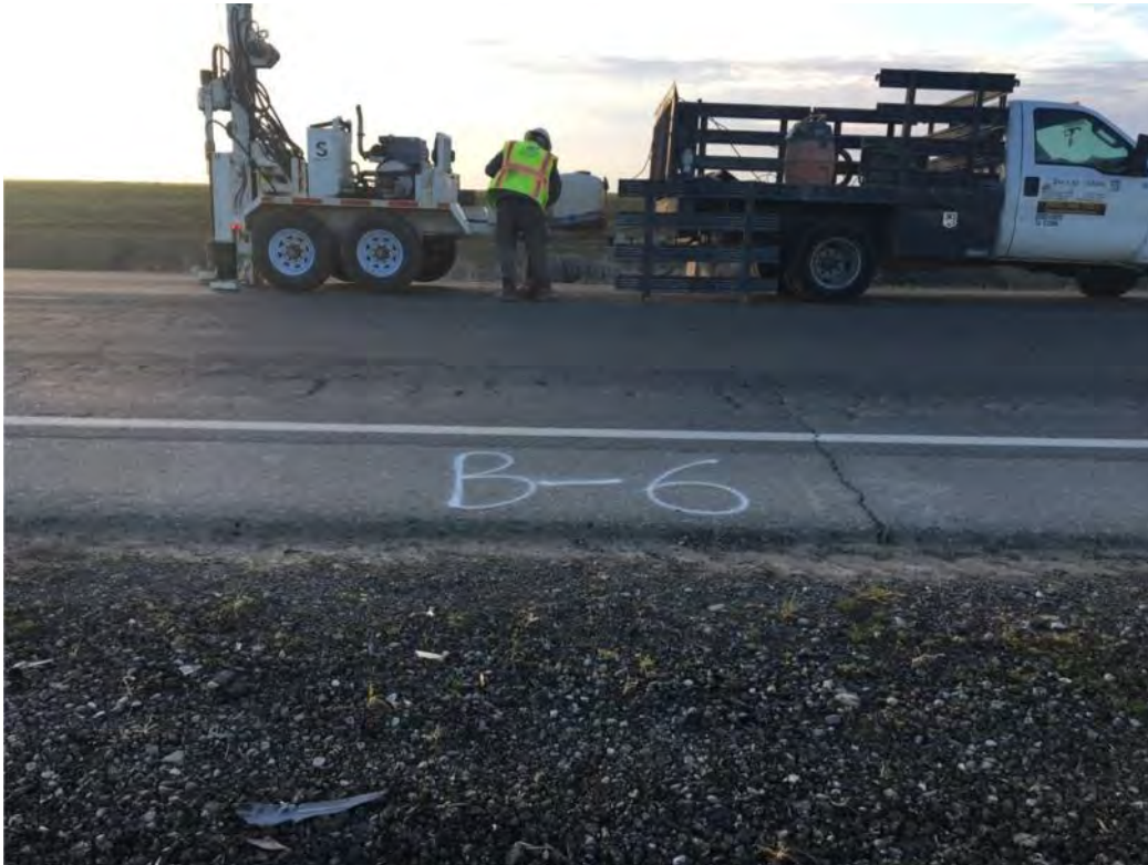
Photograph Boring Location B-6 –Note severe alligator cracking
