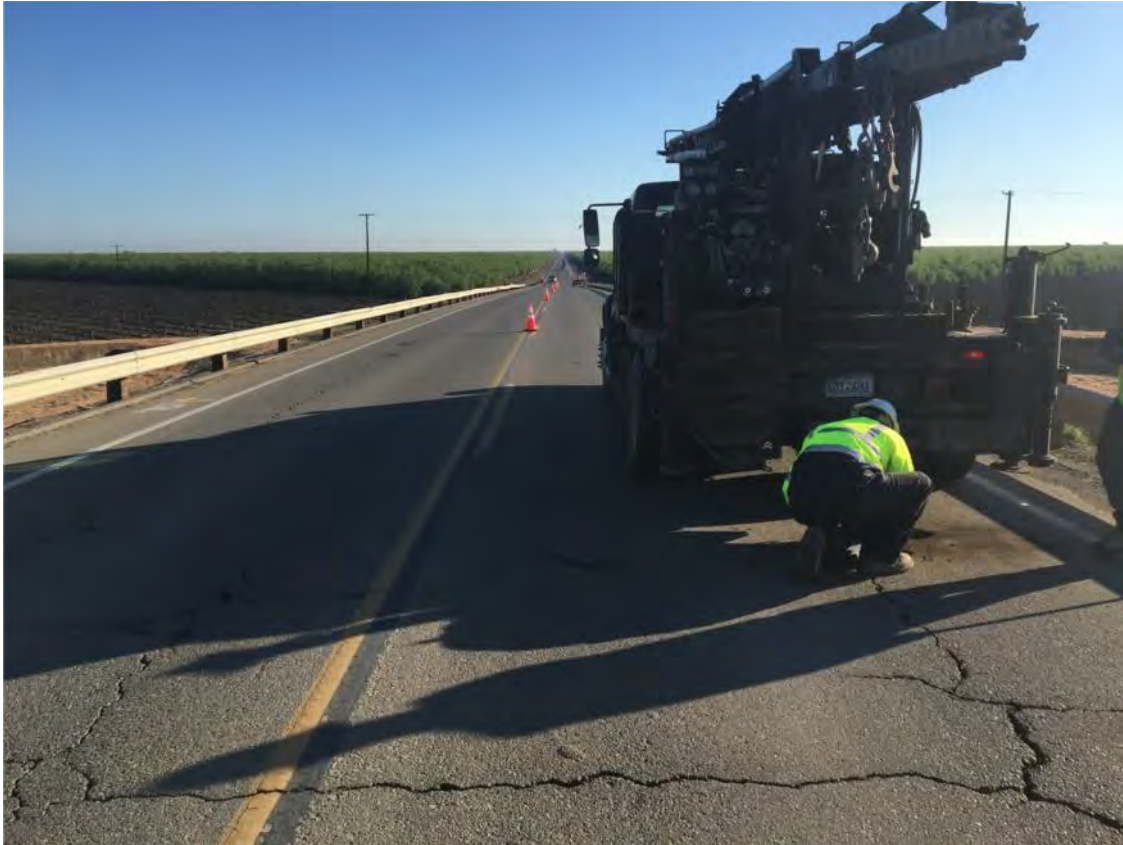
Photograph Core Location B-20 – Note alligator and block cracks
