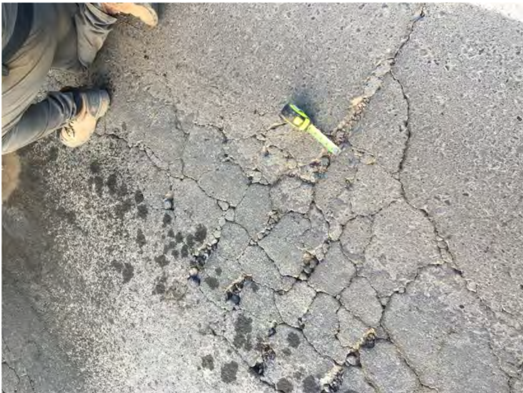
Photograph Boring Location B-7 – Note severe alligator cracking
