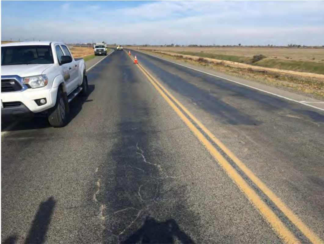
Photograph Boring Location B-1 – Note rutting and alligator cracks
