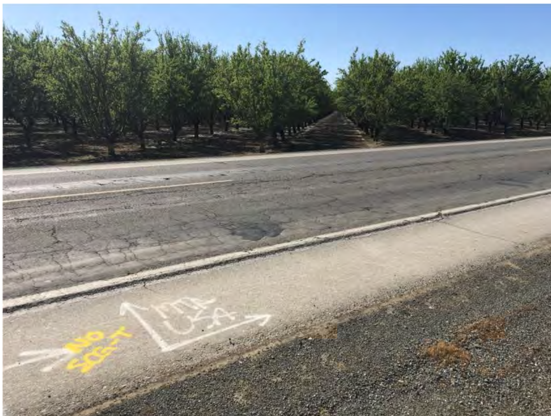
Photograph Core Location B-13 – Note severe alligator cracks, block cracks and patch areas
