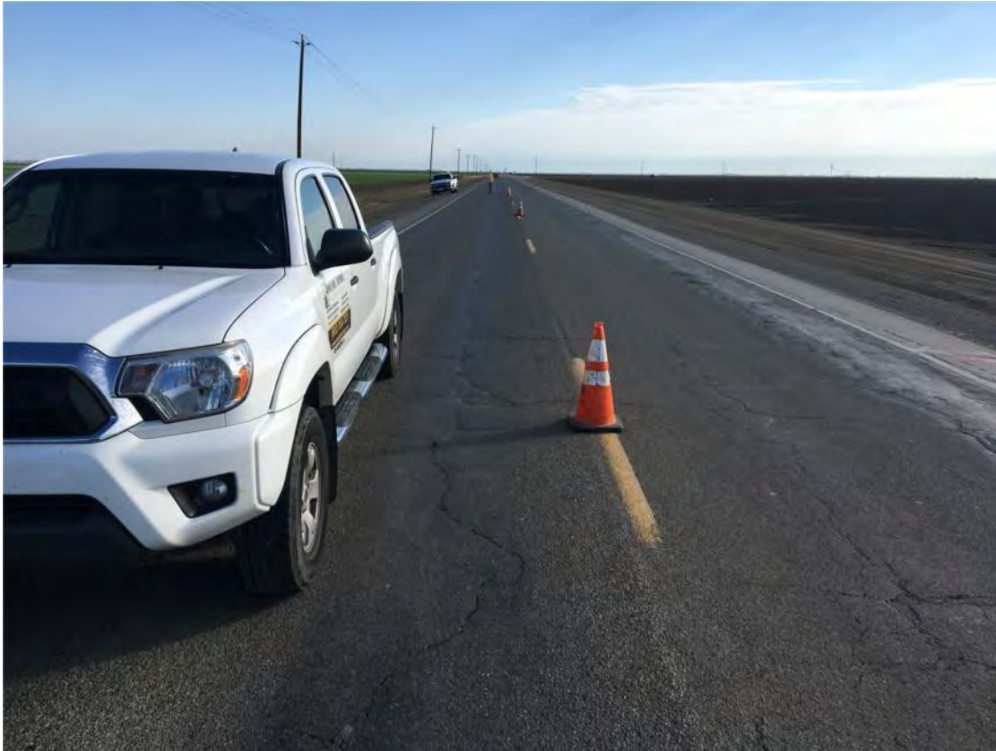
Photograph Core Location B-9 – Note block cracks, alligator cracks and patched areas
