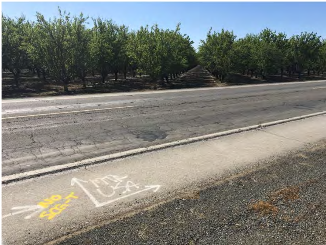
Photograph Core Location B-13 – Note severe alligator cracks, block cracks and patch areas
