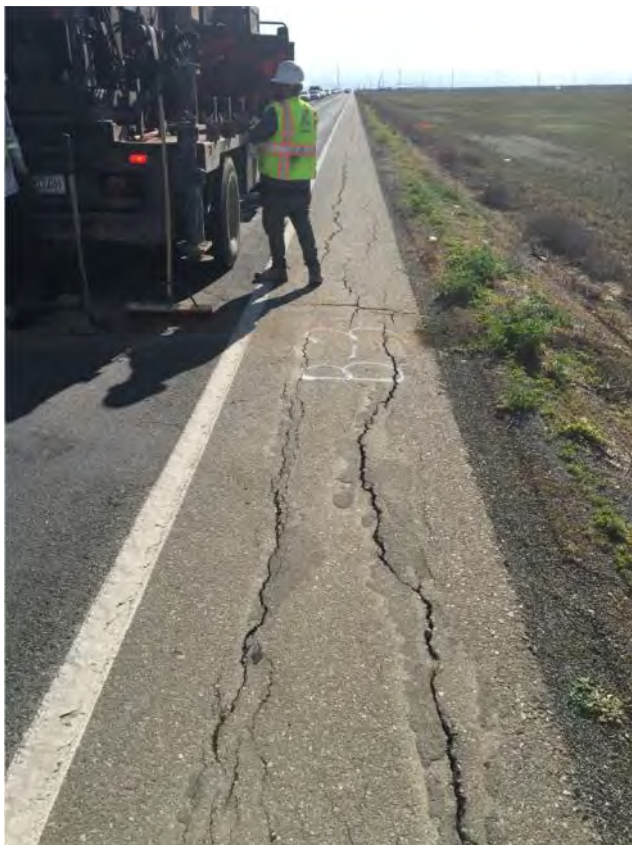
Photograph Boring Location B-3 – Note edge cracking
