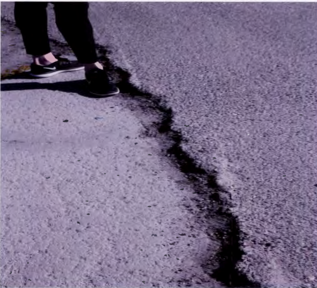
West Entrance -walking to Complex's I, II, and III 3/3/2020. Effective 5/21/2020 repairs were completed.
