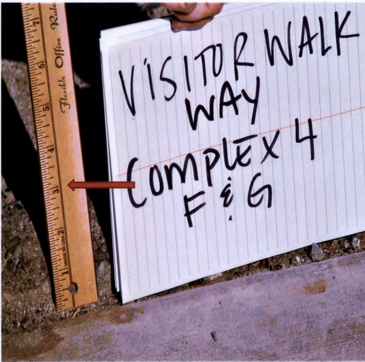
Main walkway from Complex IV going to East Entrance. 3/3/2020 Effective 5/21/2020 repairs were completed.
