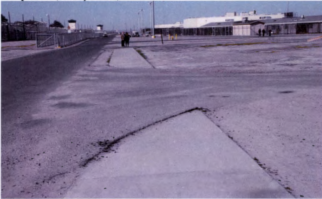
Main walkway to West Entrance from East Entrance in front of Complex III on 3/3/2020 Effective 5/21/2020 repairs were completed.
