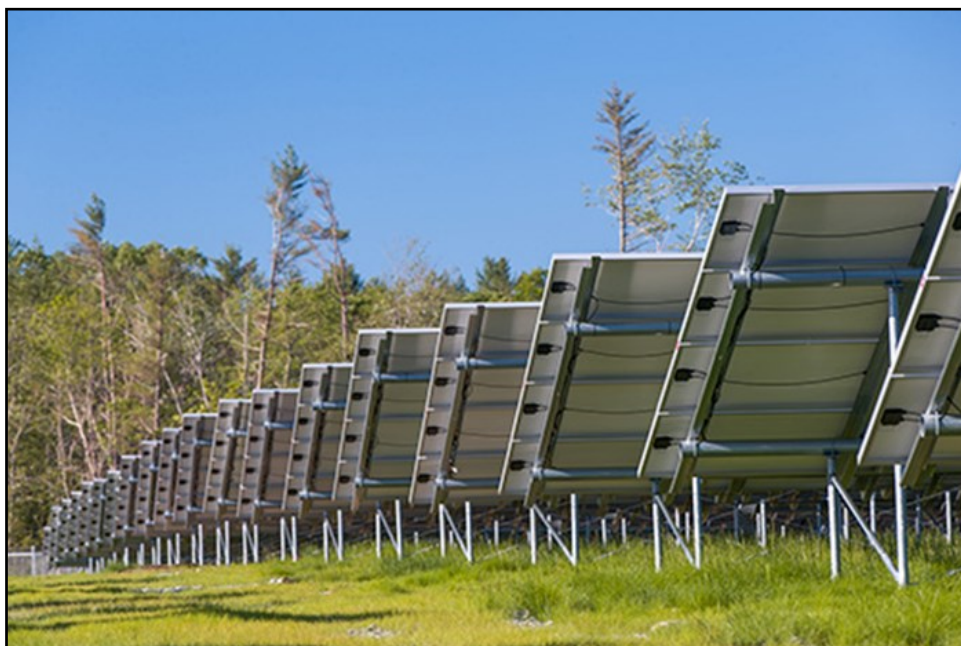
Representative Fixed Tilt Installation (Back View of Modules)
