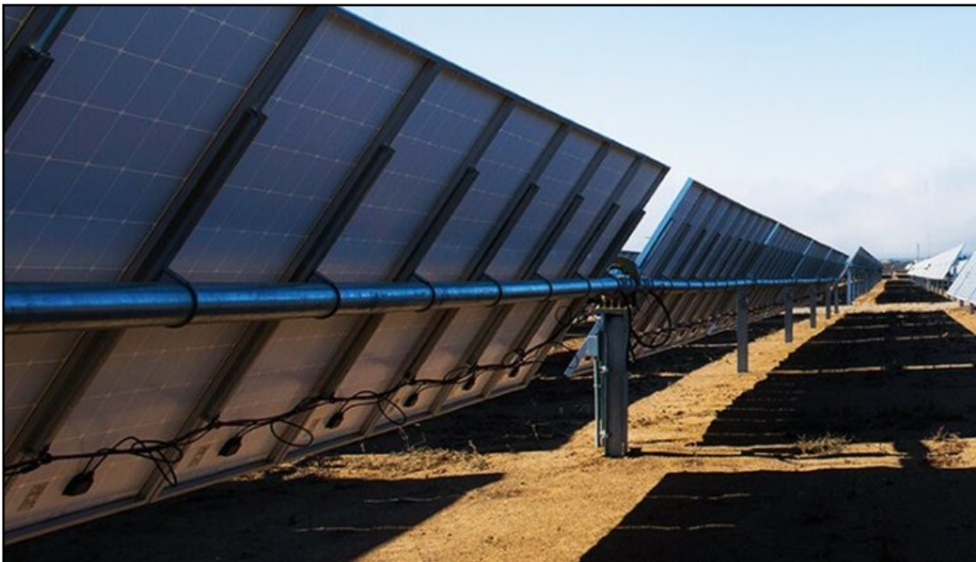
Representative Single Axis Tracker Installation (Back and Side View of Racking and Modules)
