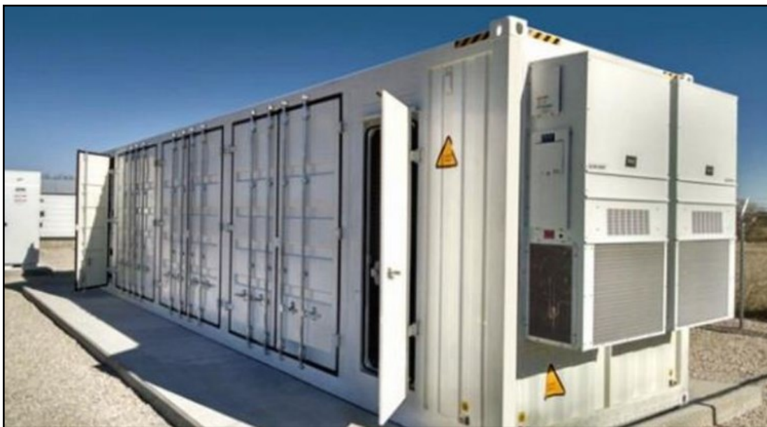
Representative Battery Storage System Enclosure (Exterior View)
