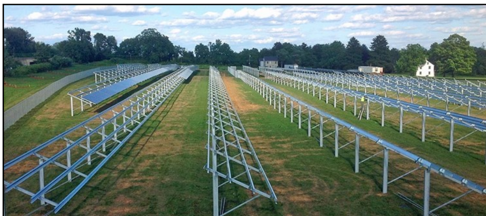
Representative Fixed Tilt Installation (Side View of Racking and Modules)
