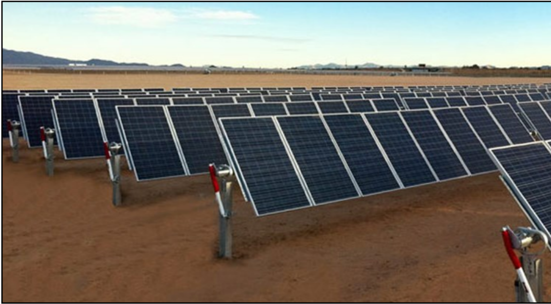
Representative Single Axis Tracker Installation (Front View of Racking and Modules)
