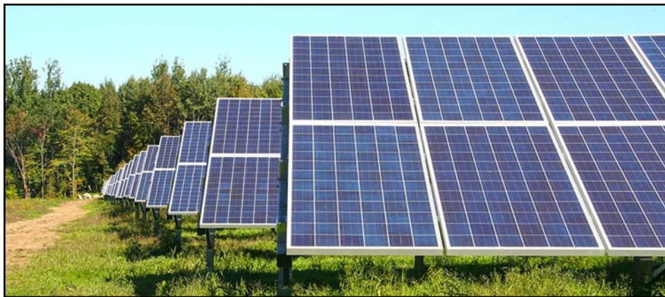
Representative Fixed Tilt Installation (Front View of Modules)
