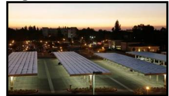
Figure AQ-9 Solar Panels
